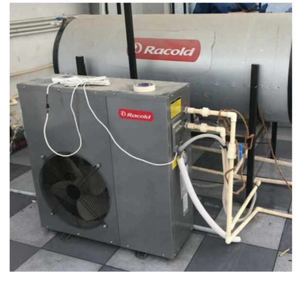
Centralized Hot Water System
